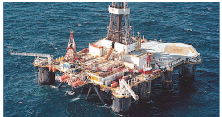
TRANSOCEAN 714, Houlder provided Engineering Services, Project Management and Construction Supervision during the rig's upgrade at Invergordon, Scotland. The scope of work included installation and integration of new accommodation modules and total refurbishment of existing accommodation.
