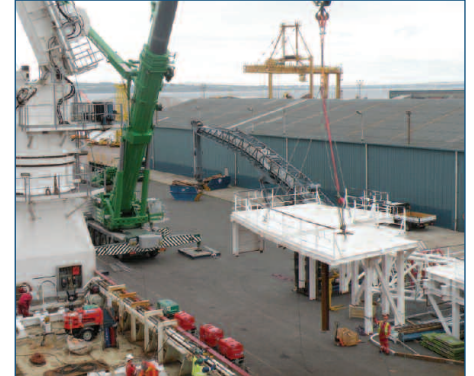
WELL ENHANCER, Houlder designed, prefabricated and installed mezzanine decking for Helix Well Ops.
