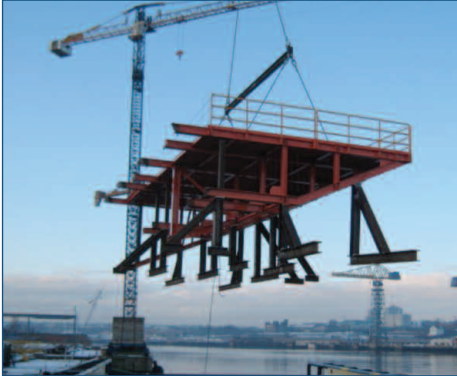
BYFORD DOLPHIN, Houlder designed and supplied this prefabricated deck extension being shipped to Norway for installation.
